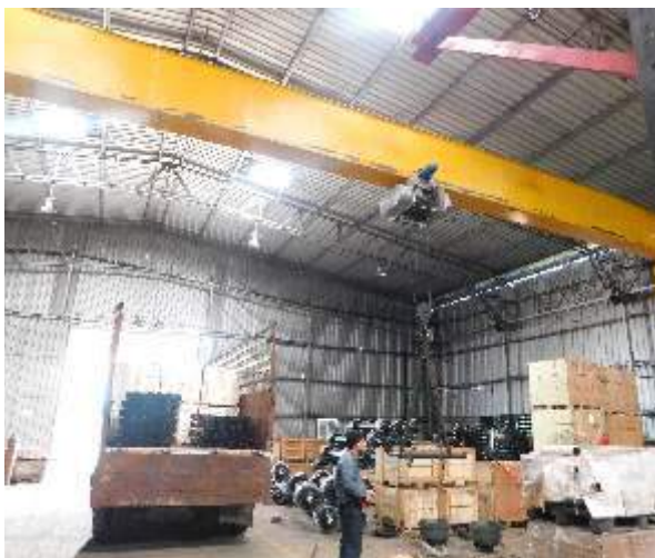
Over Head Crane
